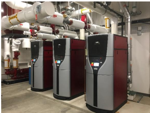
Energy efficient condensing boilers
