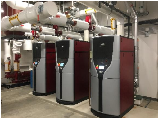
Energy efficient condensing boilers
