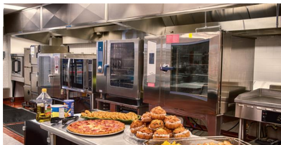
Gas powered food service equipment
